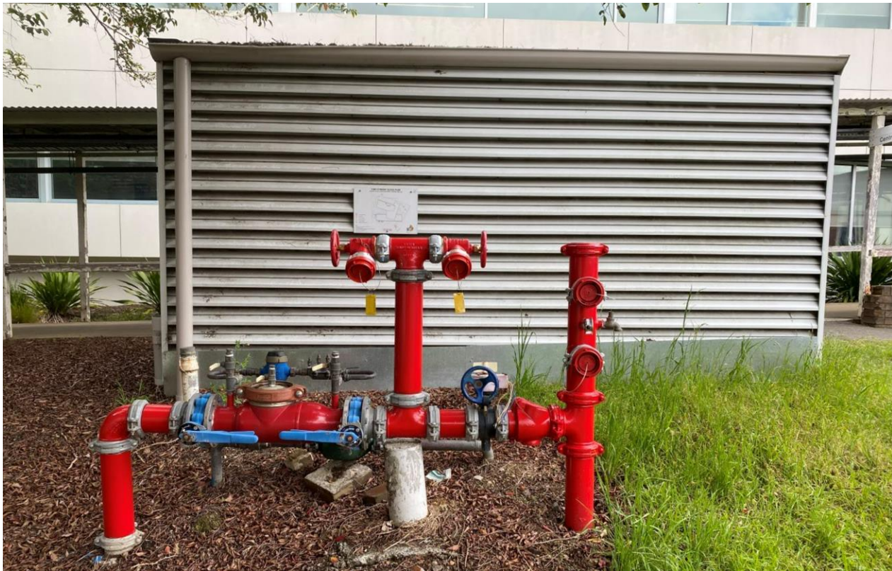
Figure 8 - FRSNW Hydrant Booster and pump-set serving building 26
